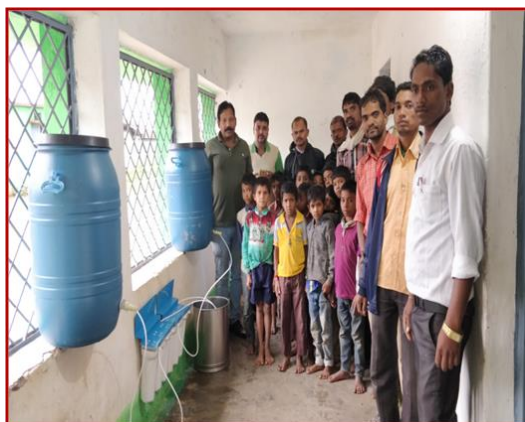
Installation of Nano alumina water filter in drinking water Rated village of Patalkot Valley the Chatravas of Chintipur village, Patalkot
