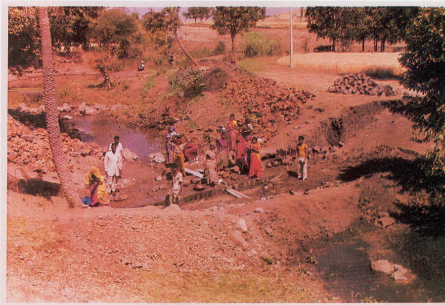
Resources Development Division was called upon to take up survey and studies in water scarce regions in Dhar district M.P. The picture shows a typical structure under construction for water conservation. (Photo Courtesy : Unicef, Bhopal)
