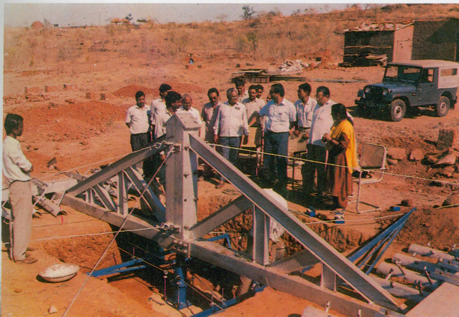
Work on plate load tests for bearing capacity of foundation soil at indoor museum site at Indira Gandhi Rashtriya Manav Sangrahalaya, Bhopal was carried out by the Building Material Characterisation Centre of RRL.
