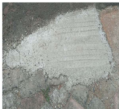
Patching on Flexible Pavement (Bitumen Surface )
