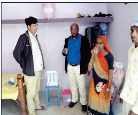
Demonstration of water filter installed in the Molukheri village of Aasta Tahsil in Sehore district, M.P.
